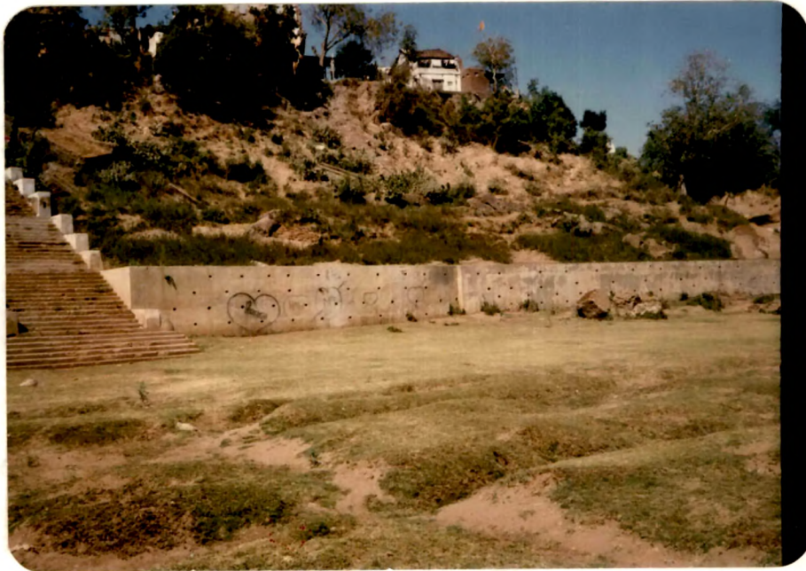
PLATE VI.1 A view of Narmada bank erosion and protection wall been constructed Loc. Sinor
